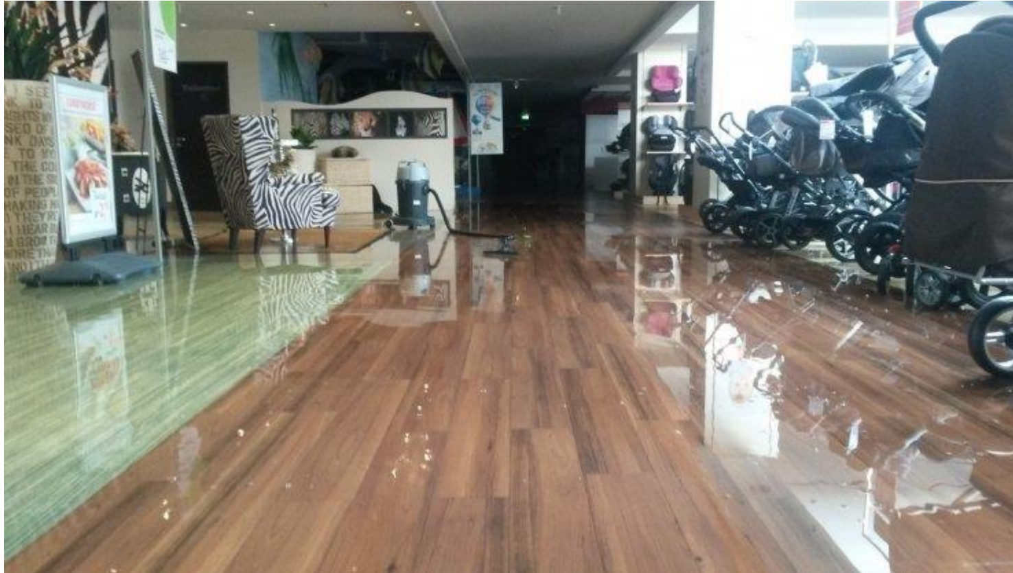
Furniture Store: Water Damage
